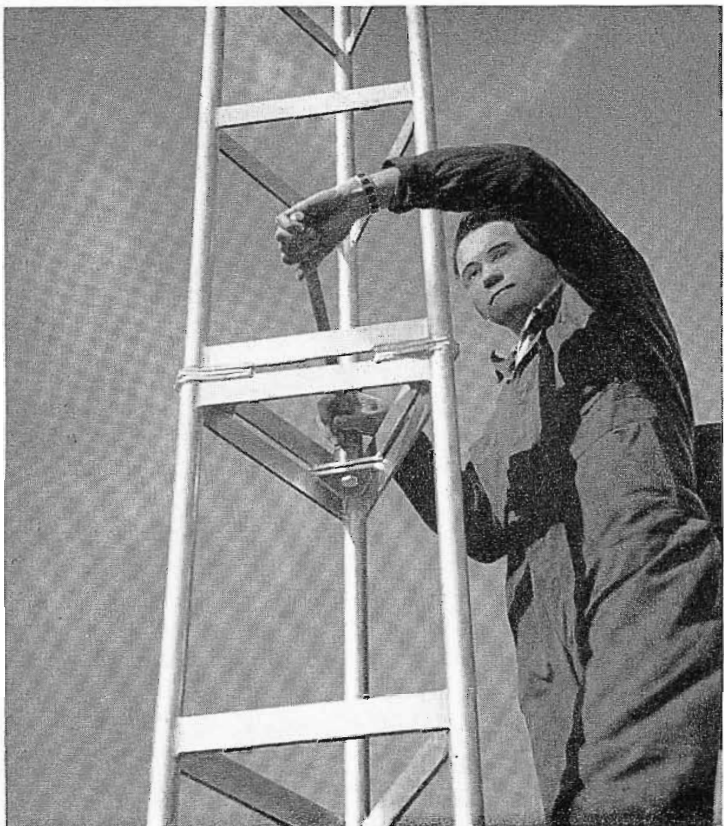
FIG. 5. Two sections of tower are being bolted together. The joint should provide electrical continuity as well as structural strength.
